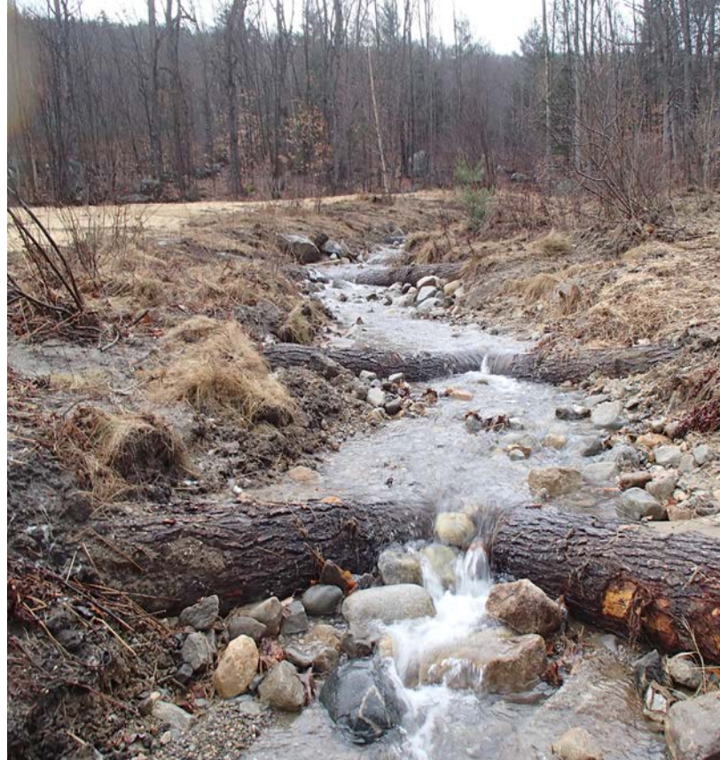
Log grade control structures during and after installation, Hebron, NH – credit: Sean Sweeney
