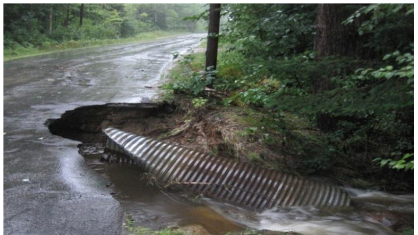
Road washout in Jackson, NH
